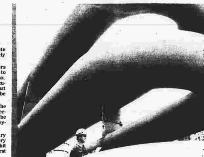
Pipe check UPI photo
